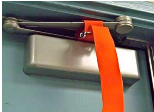
Figure 10: Strap-type Door Closer Restrictor in installed position around door closer mechanism.
